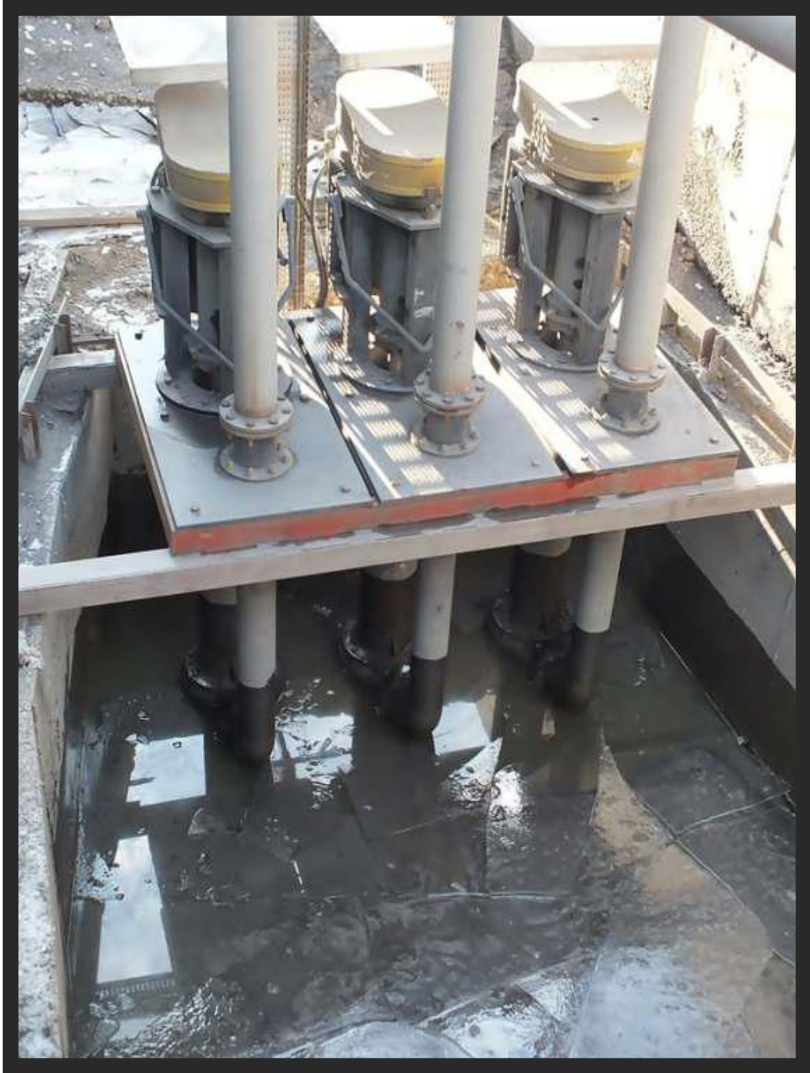
ETİ KROM CHROME PLANT (ELAZIĞ) SEP GSP KS SERIES SLURRY PUMP WITH VERTICAL SHAFT and COLUMN PIPE
