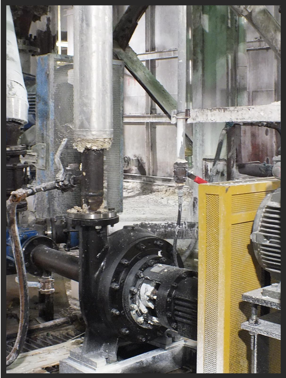
ETİ MADEN BORON WORKS (KIRKA) SEP GSP-VX SERIES HEAVY DUTY MINERAL/SLURRY PUMPS (BORON WORKS)
